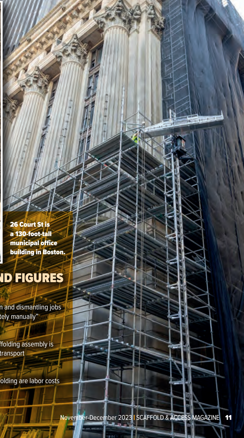
Marr began installing systems scaffolding in early June on this Boston project.
