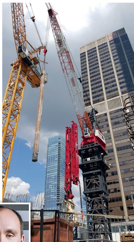
Priestly Demolition used tower cranes to remove mega columns as part of a demolition project at 1 Bloor Street in Toronto, Canada
