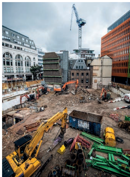
A tightly constrained site is all part of the challenge for Deconstruct UK
