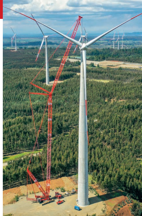
Wind energy work, including turbines and foundations, is a mainstay of activity for Burger
