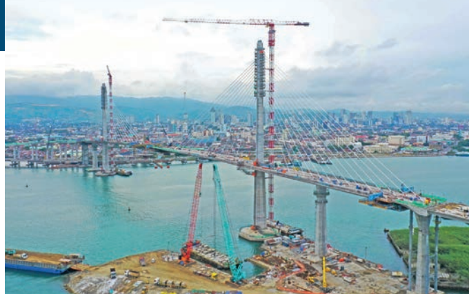
Two tower cranes from Comansa are helping to build a bridge connecting a tourist hub and international airport in the Philippines
