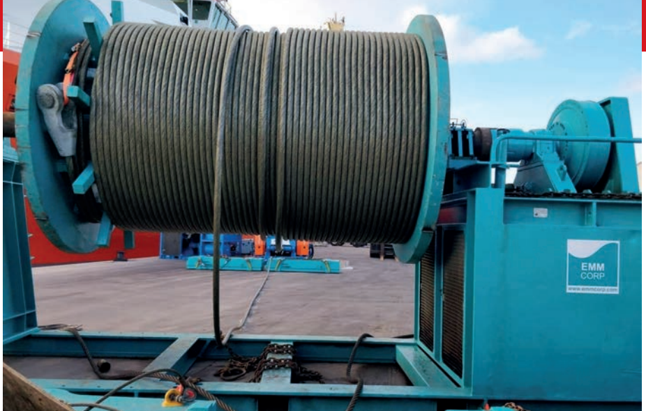
Usha Martin Group companies provided a turnkey solution for a rope replacement project
