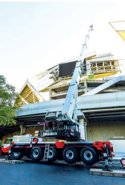
Kentucky, USA-based D CRANE RENTAL used a 150 tonne capacity Link-Belt 175|AT all terrain crane to replace video boards at the Paul Brown Stadium in Cincinnati, Ohio.
