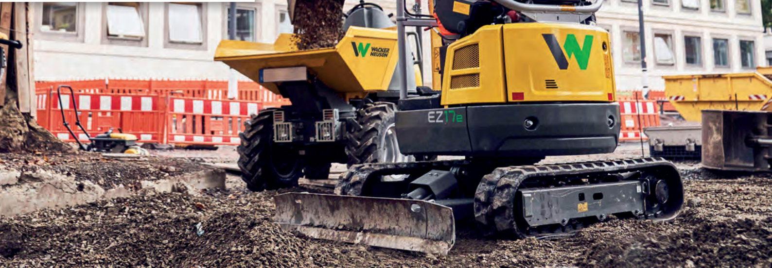
Germany: Construction company Leonhard Weiss recently tested the zero emission range from Wacker Neuson during the renovation of Stuttgart's market square. Pictured in foreground: the EZ17e Zero Tail excavator and DW15e Wheel Dumper at work.
