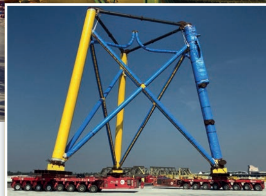
96 axle lines of SPMT was used to move the jacket pieces around, both horizontally prior to assembly and then after they had been upended
