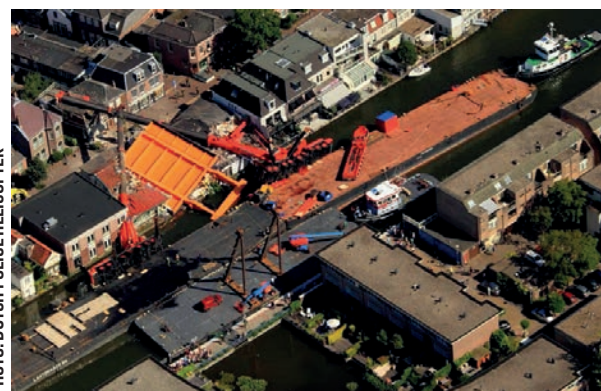
Two cranes on barges dropped a bridge deck in the Netherlands in August 2015, precipitating the ICSCA work.
