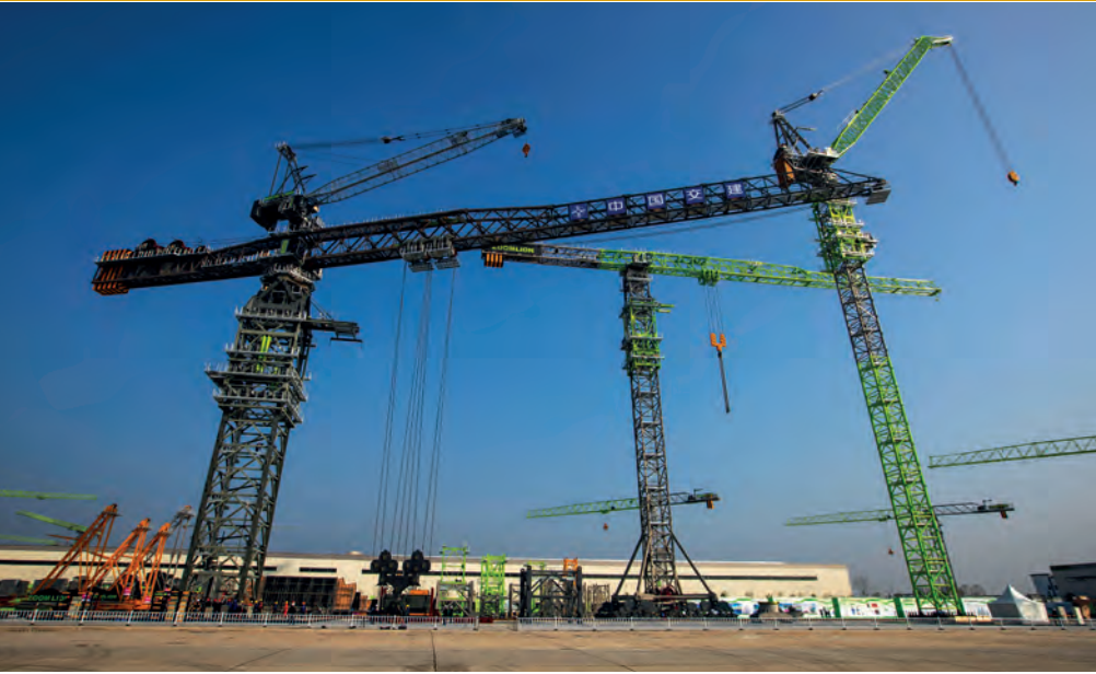
Zoomlion T1200-64W mounted on a compact 3 x 3 metre monoblock tower system for PPVC work
