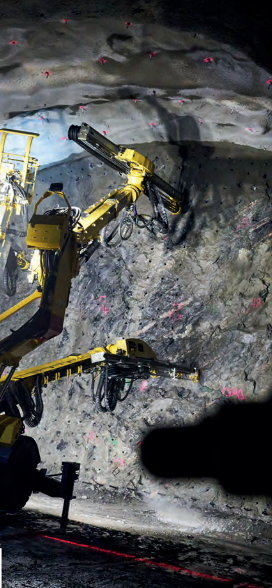
To protect the historic building above, each blast was carried out with extreme precision PHOTOS: JACOB KARSTRÖM
