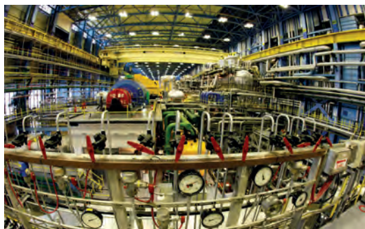
Reactor unit turbine hall at the Paks nuclear plant
