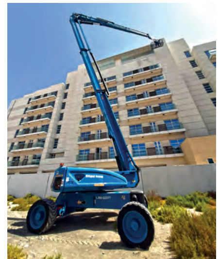
Rapid Access carrying out work in the Al Warqa area in Dubai.
