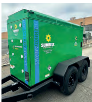
A Sunbelt battery energy storage system (BESS).
