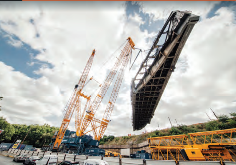
The Sarens SGC-90, a fully electric and silent ring crane, was short listed to tackle challenges and execute a project to dismantle two old railroad bridges and replace two new bridge sections.
