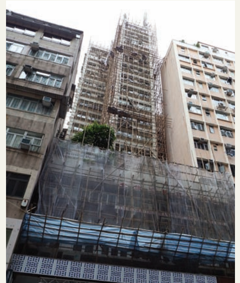
Bamboo scaffolding being used on a high rise residential building in Hong Kong.
