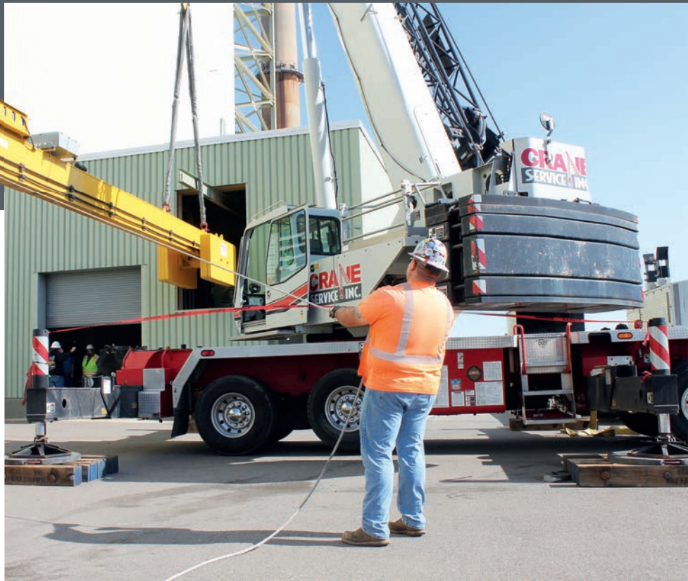
The engineered solution was to use a cantilever lifting beam rigged to a 100-ton capacity Link-Belt HTC 86100 truck crane to remove and replace a critical drive motor.
