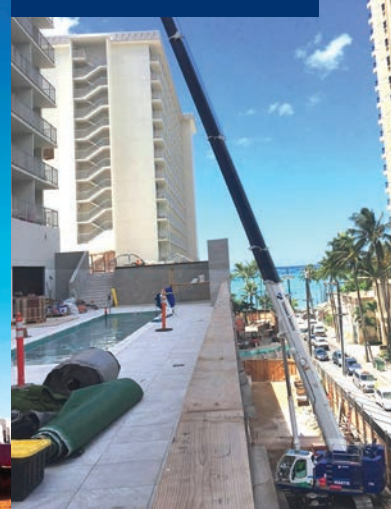
CONFINED JOB SITE
