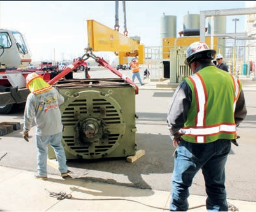
The drive motor was rigged to the cantilever lifting beam with four 17-ton shackles and four 8-foot endless slings in a basket.
