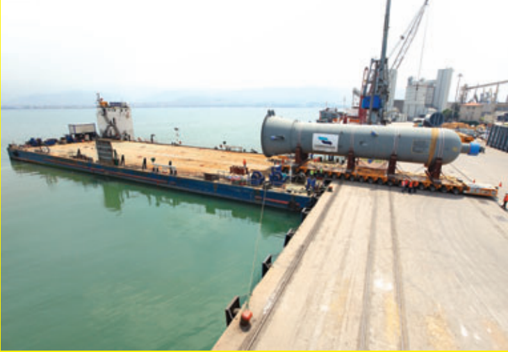
Transportation of 918 tons Reactor from Derince Port to Tupras Refinery by 20 axles 4 file Goldhofer PST/SL-E trailer on the barge.
