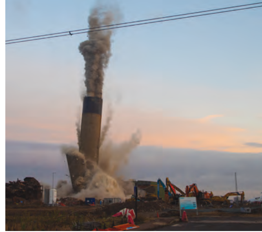
Brown and Mason proposed a vertical collapse mechanism for the Littlebrook chimney
