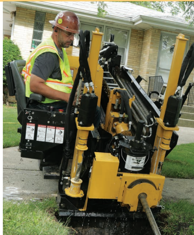
Directional drilling rigs are one of the least invasive tools for installing conduit underground
