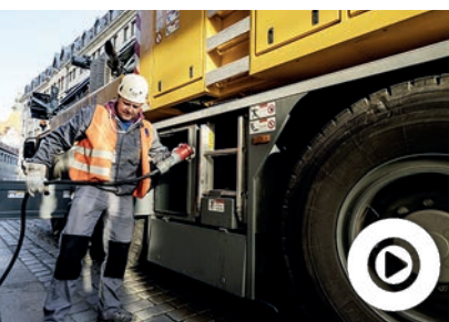
Mains site power allowed the crane to work almost silently in Dresden's historic old town and without engine exhaust emissions
