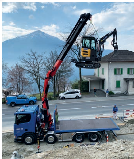
Swiss application for a Palfinger PK 37.002 TEC 7 delivering construction equipment for Rust + Co
