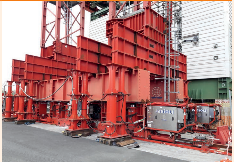
The Fagioli stacking and de-stacking operations were operationally executed in 24 hours for each single activity after a month of ground preparation and equipment assembly
