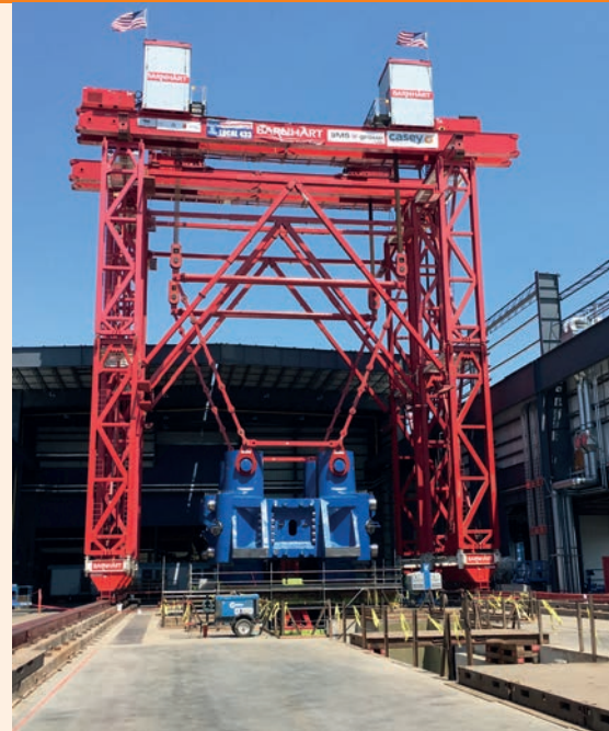
Barnhart's press assembly project comprised 3,500 engineering hours and over a year of planning
