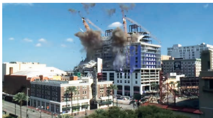
Moments after ignition of the explosive charges to bring down a pair of tower cranes after the partial collapse of a hotel during construction
