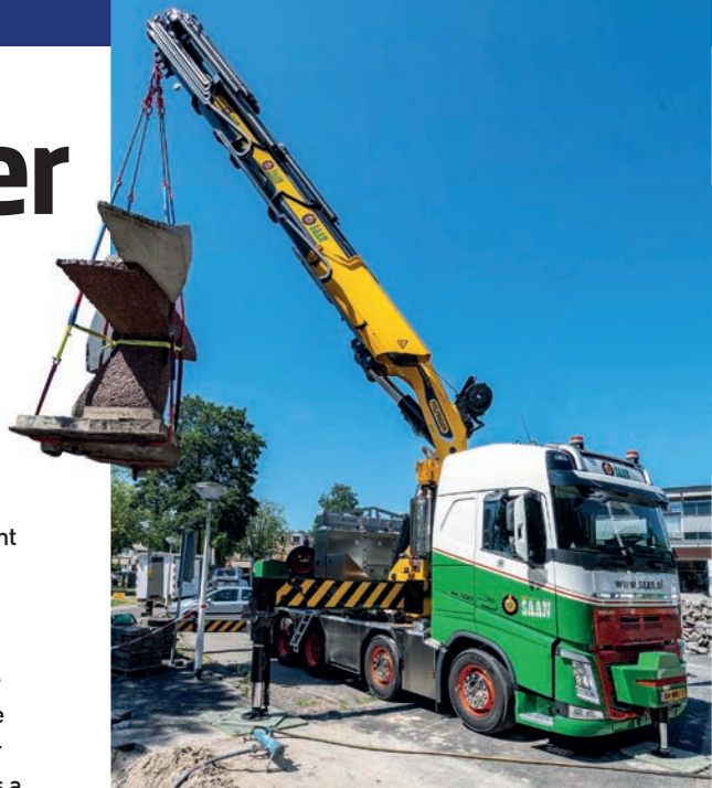
Koninklijke Saan's new Volvo FH 500 10 x 4 with Palfinger PK 165.002 TEC7 crane out at work
