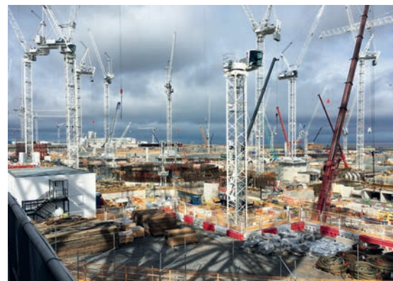
55 tower cranes will be on site, all fitted with anti-collision systems from AMCS
