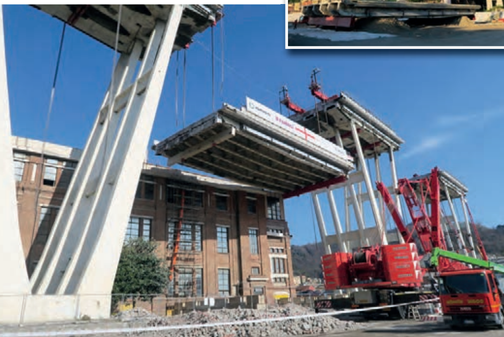
(Left and inset) The first section makes its descent of nearly 50 metres to the ground suspended from four 600 tonne strand jacks
