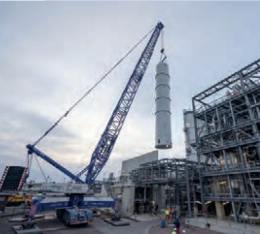
Maxikraft used its Liebherr LTM 1500-8.1 and LTM 1750-9.1 mobile cranes to hoist the tank
