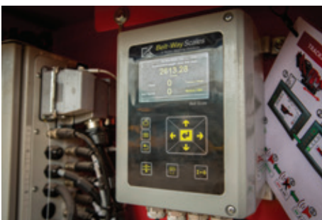
T link allows plant to be monitored remotely
