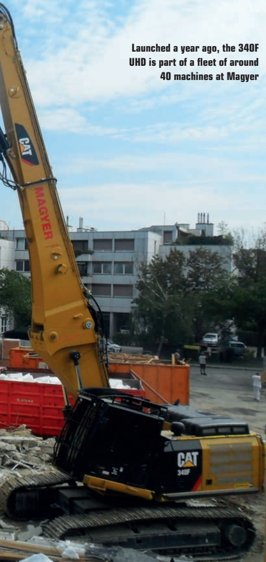
View from street level of the Wolkersdorf elementary school, with the demolition project in the background
