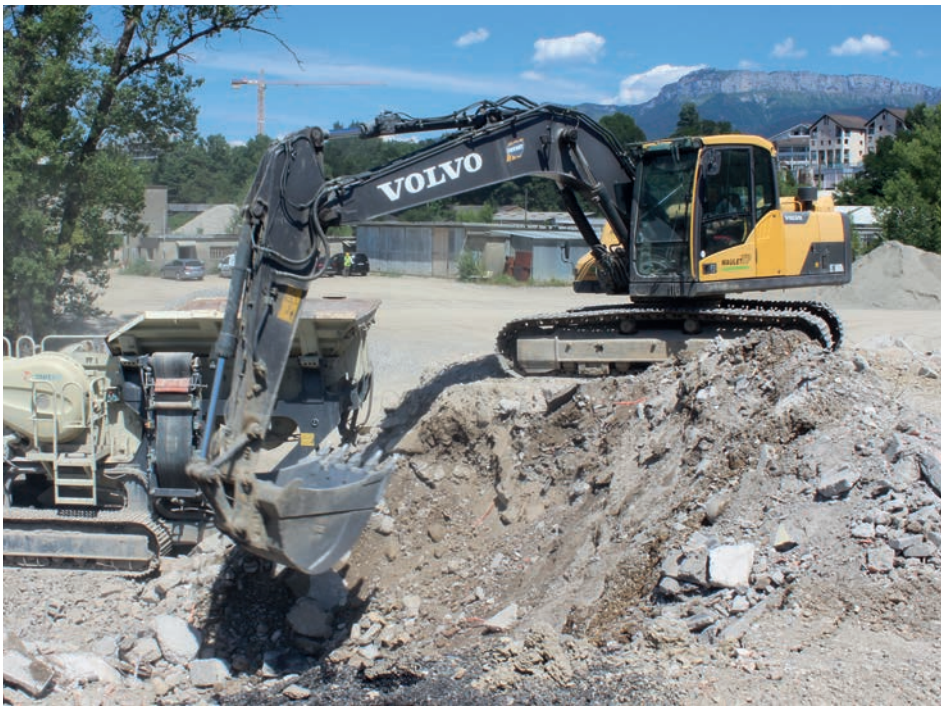
The LT96 in tandem with a Volvo EC1600L excavator. Distributor Groupe Payant is active throughout France
