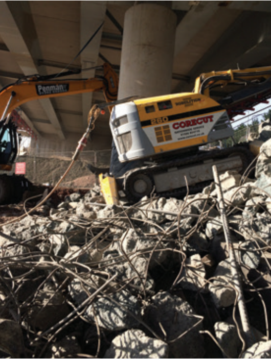
Controlled demolition of the existing BP Pipeline protective slab by Hydraulic Bursting and Robolition
