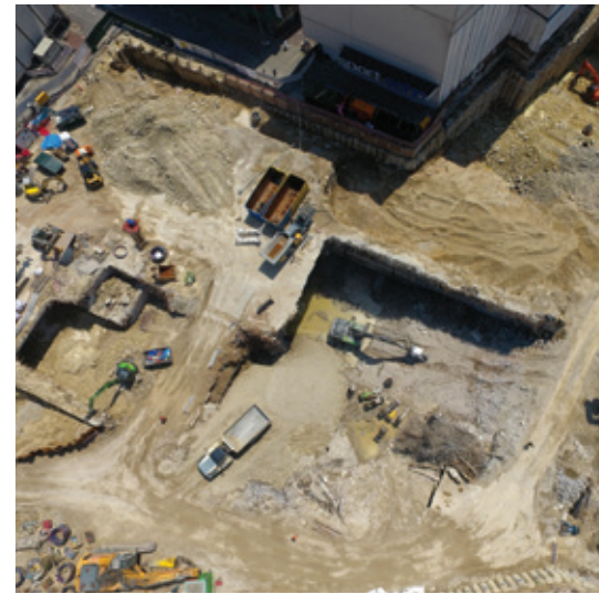
The Sedelhöfe site in Ulm, Germany, contained numerous old buildings that had to be demolished
