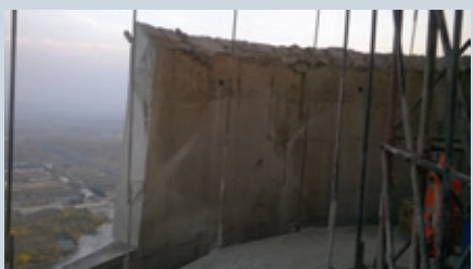
Tyrolit said that controlled deconstruction was the only option available for the 250 m high chimney
